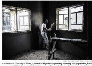
BOUNTY The city of Warri, center of Nigeria's burgeoning economy and population, is undergoing a building boom, including the opening of the city's first mall last spring. Page 2
